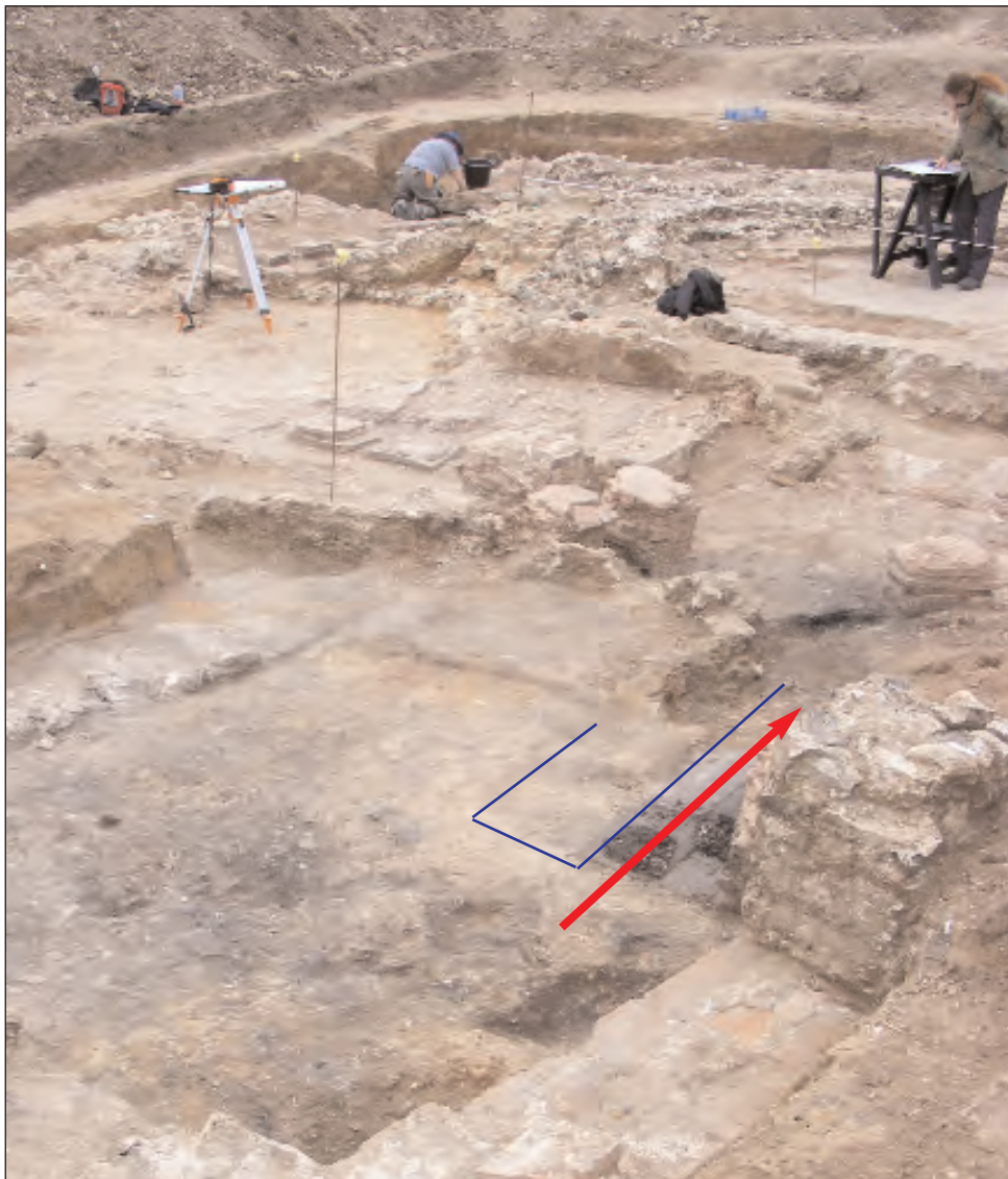
Fig 37. The furnace room (Room 2) on the north-east side of the octagon building had been built later than the main building, but how much longer is impossible to say, it could be as little as a week. In the photograph (left) the red arrow shows the direction of hot gases from the furnace into the main octagonal building. Still discernable is a 'flume' of ash flowing into the underfloor hypocaust system of Room 1. The blue line rectangle indicates the position of the left-hand side furnace wall. Joining the two walls would probably have been a brick arch supporting water tanks which could have provided hot water for the bathers.
